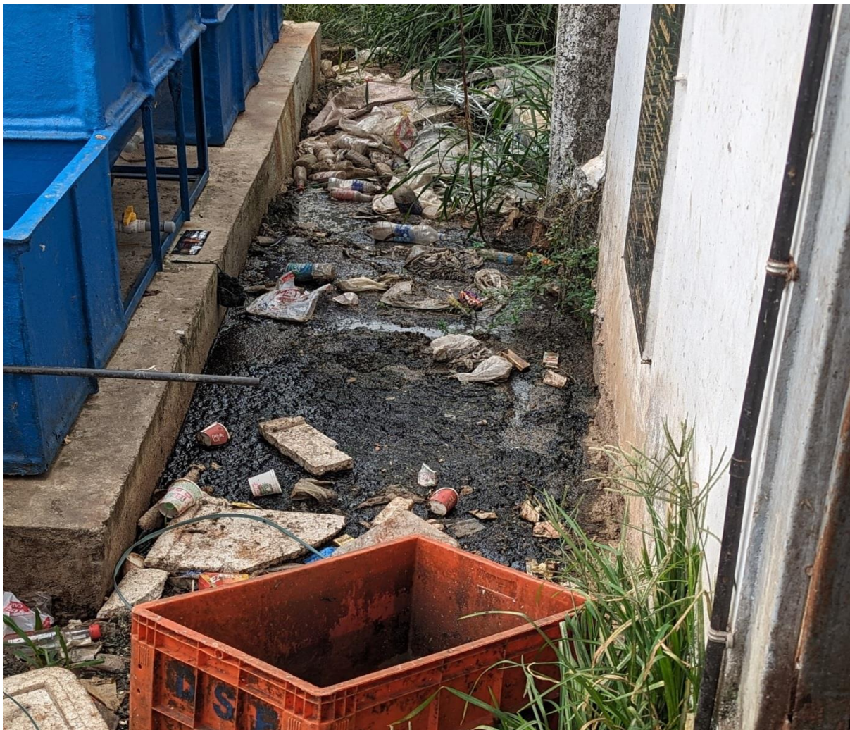
Untreated waste water is being deposited directly to the land
